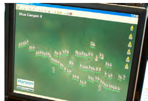
SCADA system computer.
